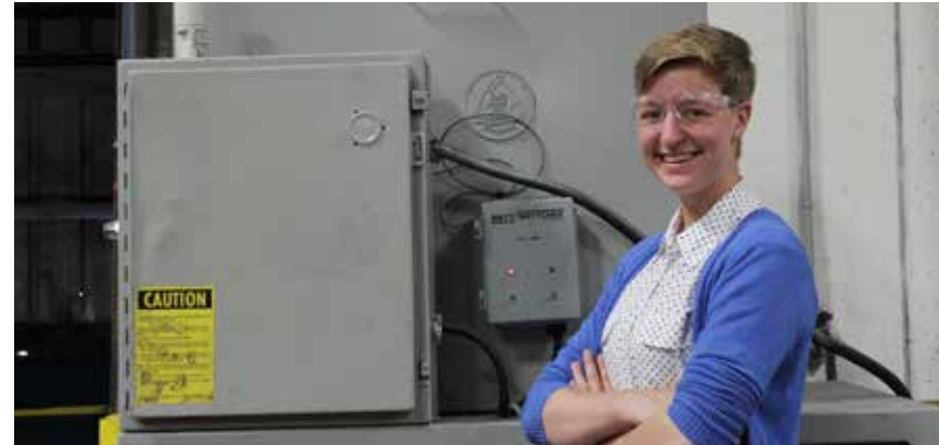
Emily Daniel from MnTAP with the Watt Watcher™ granulator controller installed at Plastech in 2016.
