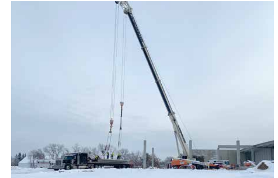
Workers attach cables to a concrete wall section to be hoisted into place for Plastech's new addition on December 19, 2022. The temperature was below zero at the time and didn't get above zero all day.
