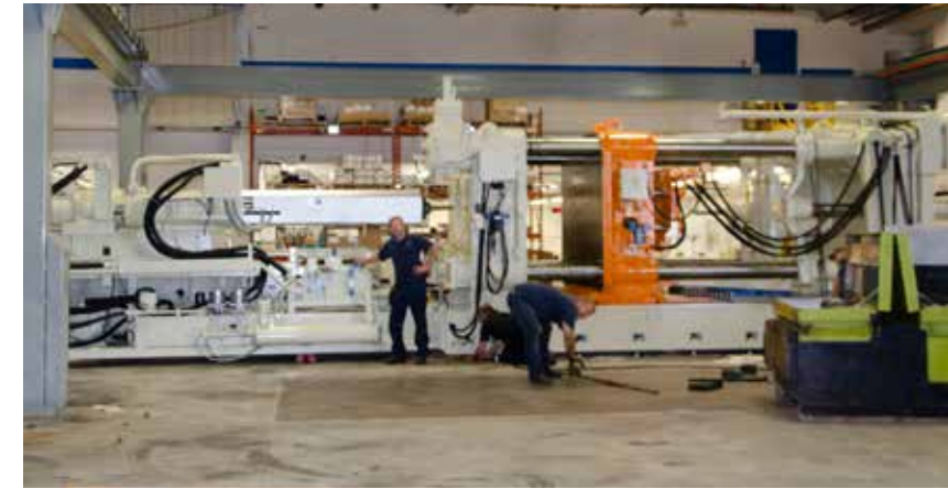
Millwrights from Quickway Rigging setting up the new press on its reinforced concrete floor.
